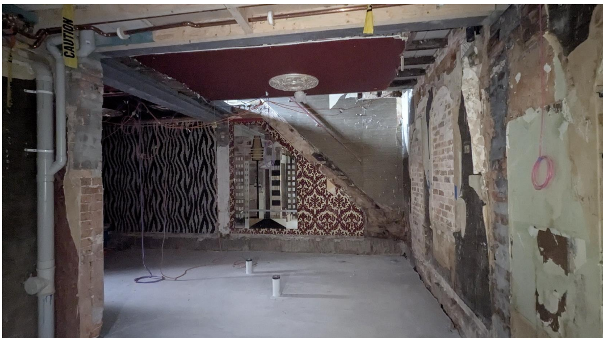
Figure 7: The current stripped and vacant condition of the interior of the premises (being the ground floor level of 101 Albion Street)
